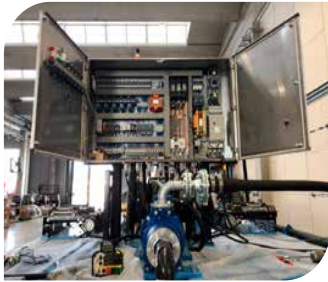
Electric control panel
